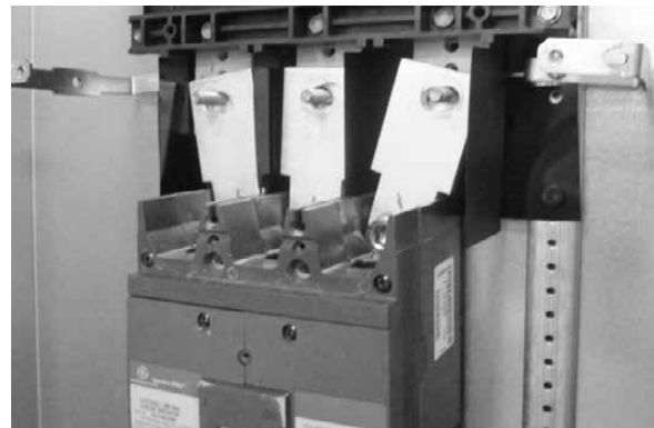
Figure 6C. Illustration of phase barrier correctly aligned between main bus bars and connecting straps.
