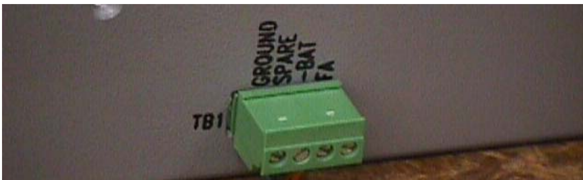
Figure 1-4. Input Power Connection
