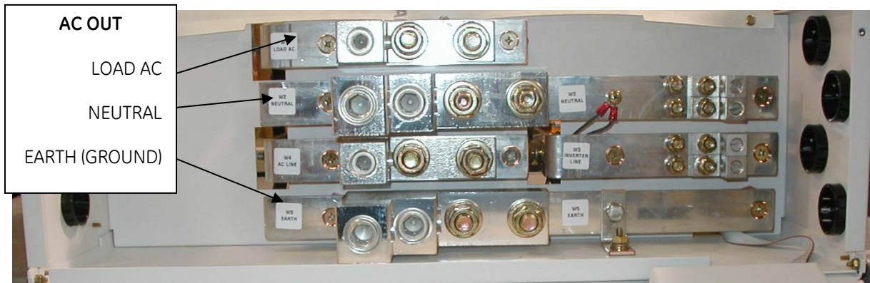
Figure 3-5: Load Connections from Maintenance Bypass Panel
