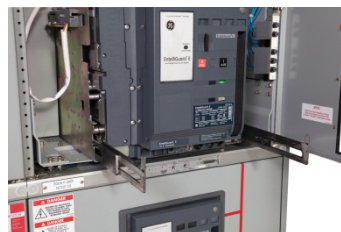
Figure 3.6. Circuit Breaker in DISCONNECTED Position
