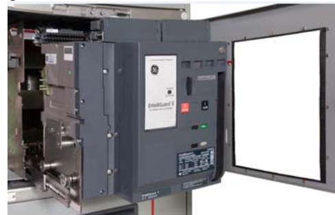
Figure 3.11. Circuit breaker Pulled Out of the Cassette for Unloading
