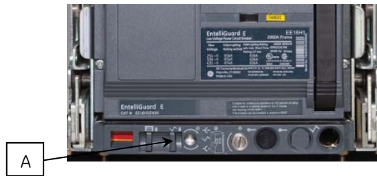
Figure 5.2. Circuit Breaker Security Padlocking Location
