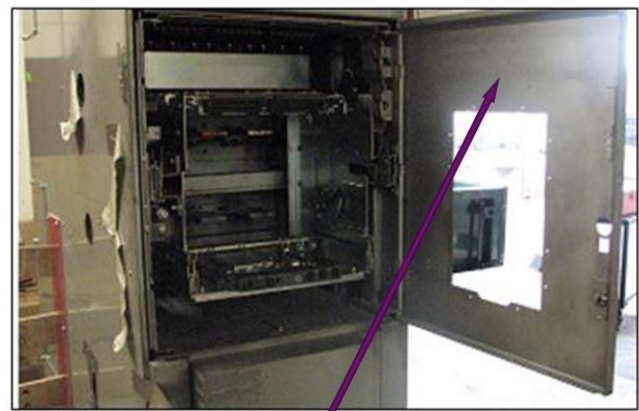
Figure 30. Cabinet with Compartment Door Open
