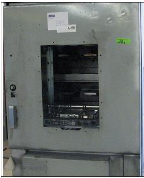
Figure 29. Cabinet with Compartment Door Closed
