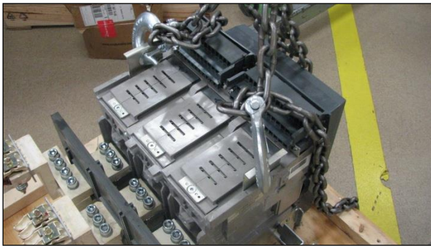
Figure 8. Crane Lifting Hooks Can Damage Lifting Holes and Ears
