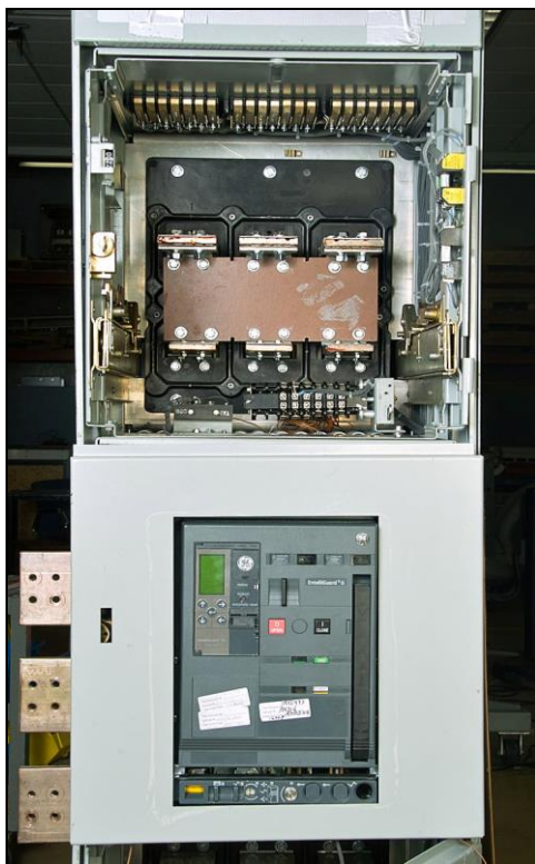
Figure 6. AKD6 Breaker Compartment (Upper and Lower Compartments)
