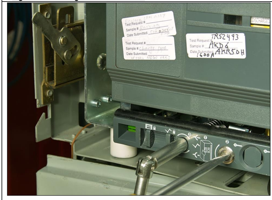
Figure 25. Racking in AKD6—Retrofill
