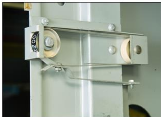
Status indicator (connect/disconnect) is a leftover device from the legacy breaker. Although it does not interfere with the retrofit, this mechanical indicator can be removed, if desired.
