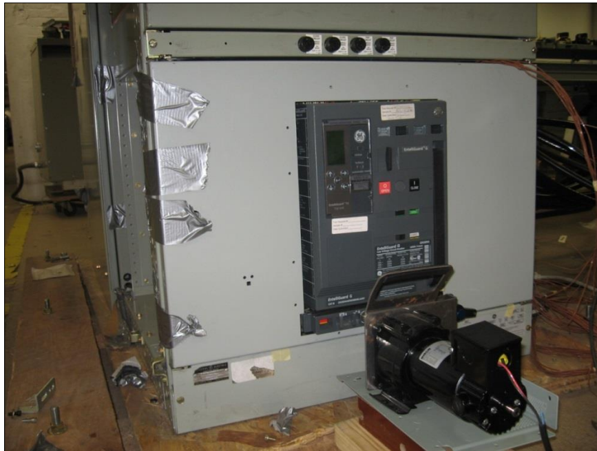
Figure 16A. Remote Racker Assembled to Retrofill in AKD-8
