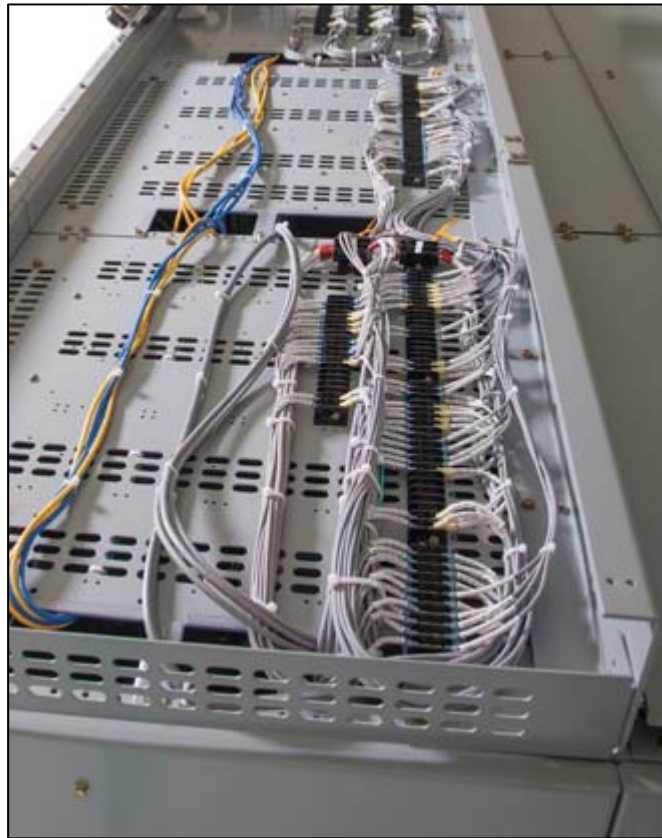
Fig. 4-14. Interconnect control wiring and Ethernet cables in the wiring trough on top of the equipment
