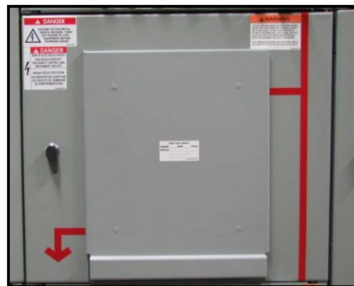
Fig. 7-4. Future-use breaker compartments
