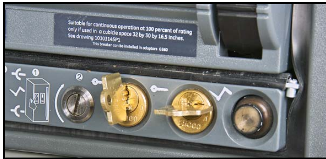
Fig. 7-5. View showing circuit breaker key interlock to provide protection against unauthorized operation
