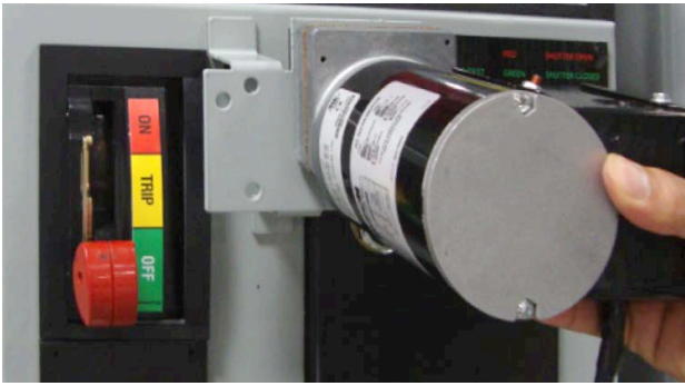
Figure 3. Mounting motor on door
