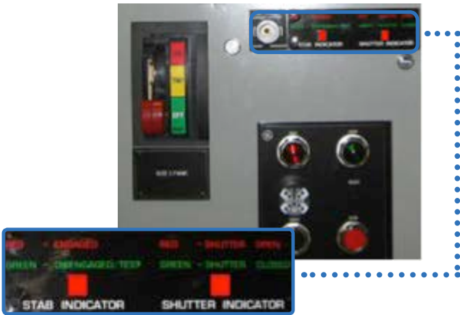
Figure 7. Mechanical indicators showing ENGAGED condition
