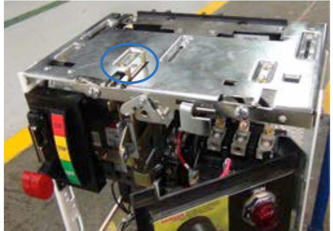
Figure 8. Stab and unit interlock shown extending through the top of the top plate
