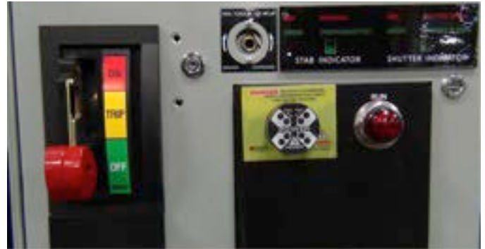
Figure 5a. Lead screw accessible in disconnect “OFF” condition
