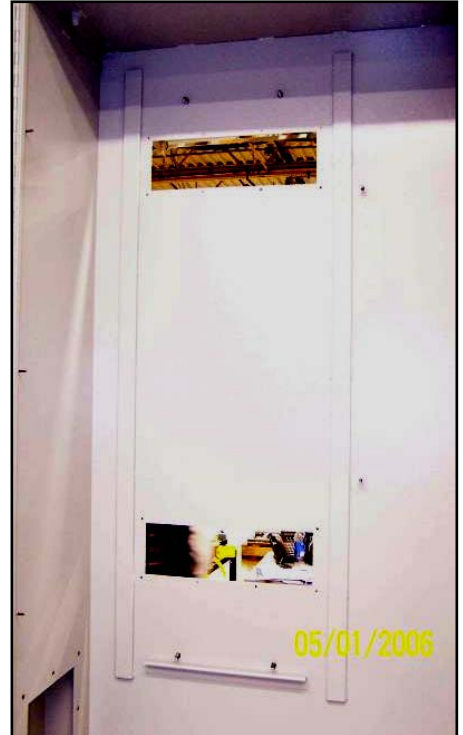
Figure 7. Back interior wall of enclosure with cutouts and hardware
