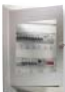
Room distribution panels
