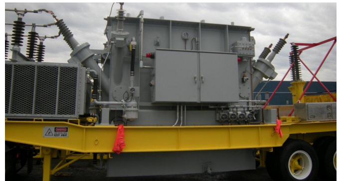
1966 30 MVA GE Mobile Substation as remanufactured.
