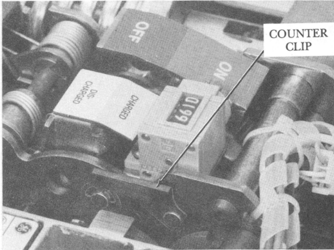
Figure 3. Mechanical counter installed in breaker.
