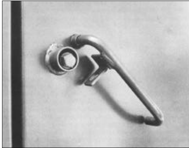
Low-voltage door handle. Padlock cannot be engaged until bolt is seated.
